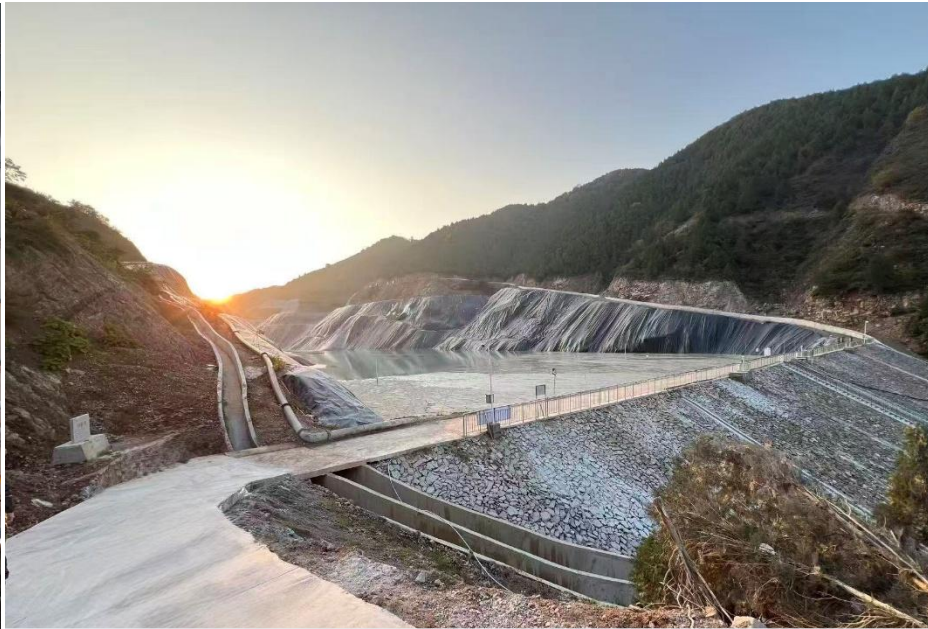
TSF No. 3 Supports LOM Production and Beyond
