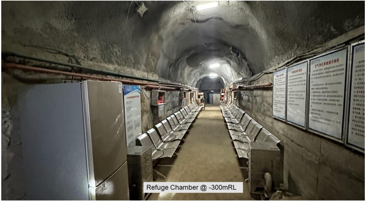
Figure 16.11: Permanent Refuge Station at -300mRL
