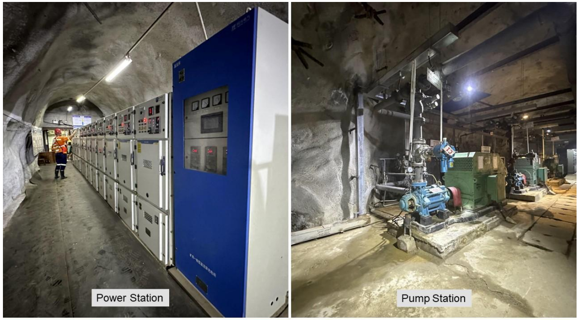
Figure 16.9: Pump and Power Stations at -300mRL
